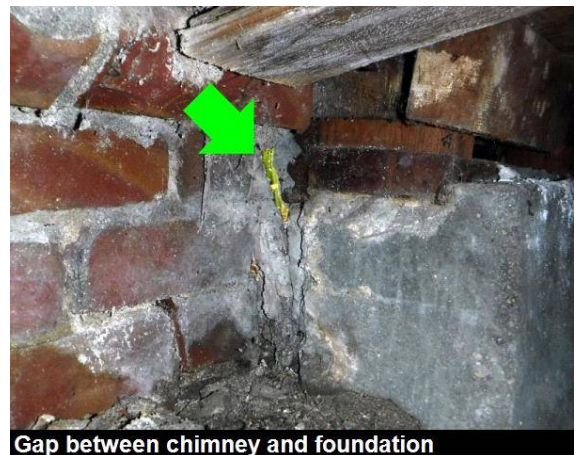
Gap between chimney and foundation
