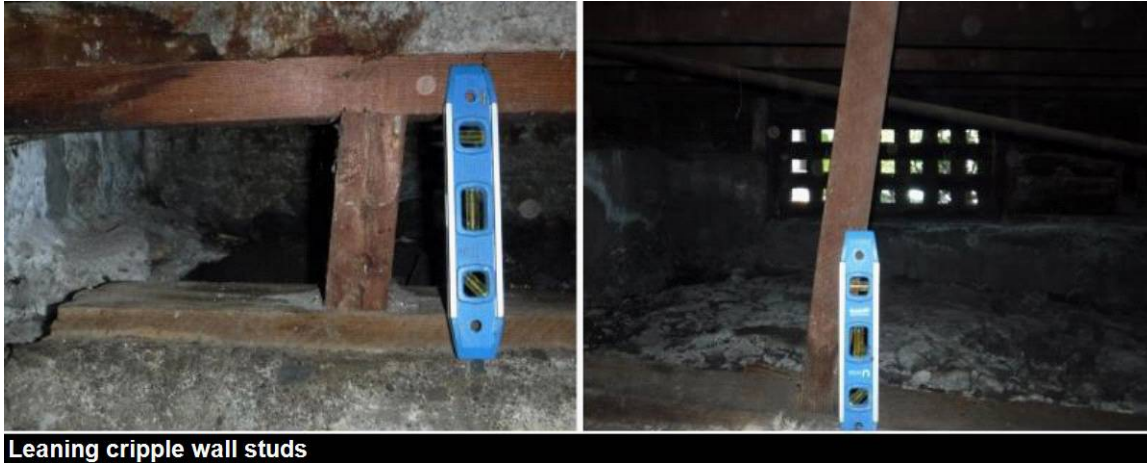
Leaning cripple wall studs
