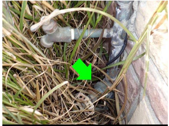
Main water valve
